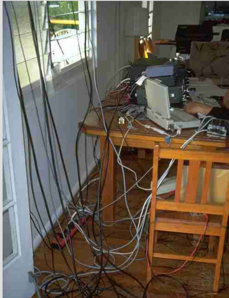
9Y4NW: Indoor cabling
